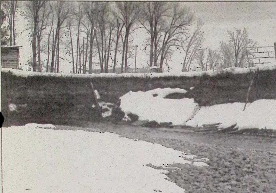
Area of Allison Creek where the embankment and stackyard fence washed away last year.
