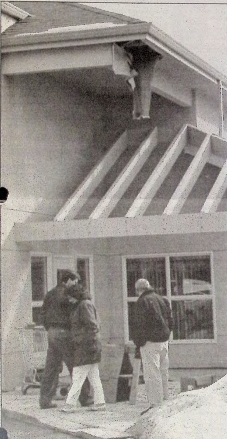
Community Services Administrator Joyce Fraser, center, spent most of February 17 with B.C. Housing officials inspecting damage to Vermillion Court and the probable cost of repairs. B.C. Housing will foot the bill. Note the stucco falling away from the roof of the 6 month old building.
