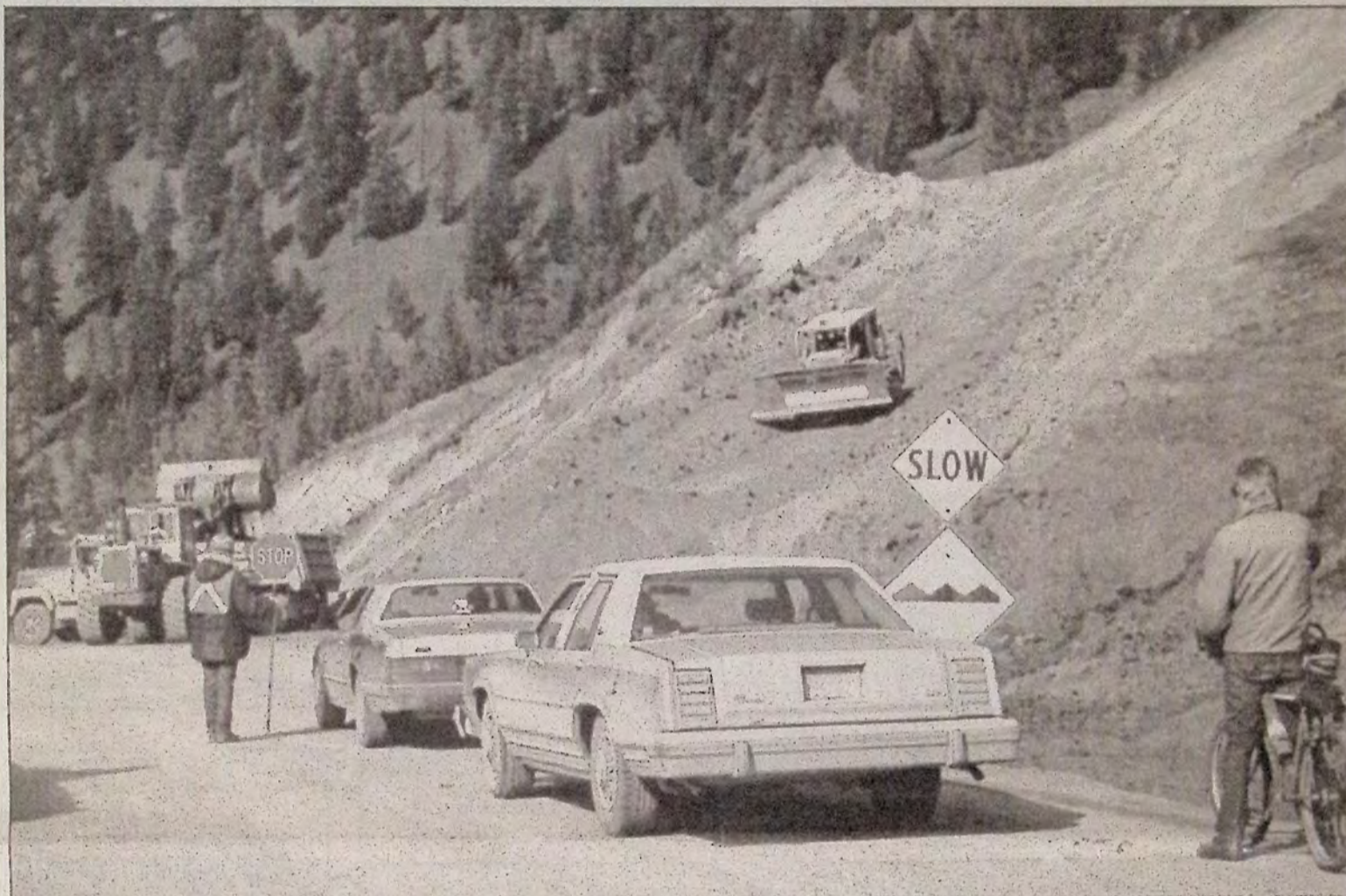
The reconstruction of the collapsed area near Peterson Bluffs on the Tulameen Road is well under way. Above, Linda English flags traffic as Jim Thomas pushes road - building material to be loaded into dump trucks. Controlled traffic will continue until the project is complete.
