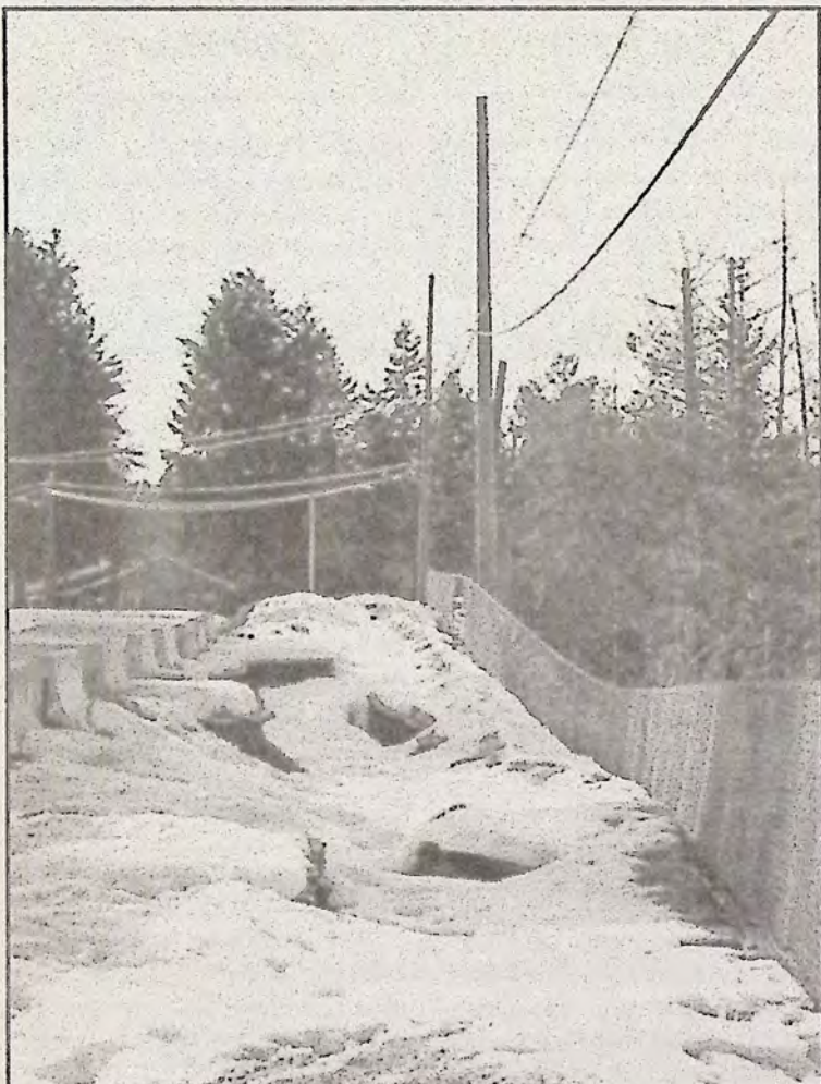
The sliding concrete retaining wall on Mayne Avenue continues to be a problem with no solution in sight. Road reconstruction is necessary and expensive, and Town Council has insufficient funds for the project. Provincial coffers offer Council nothing.
