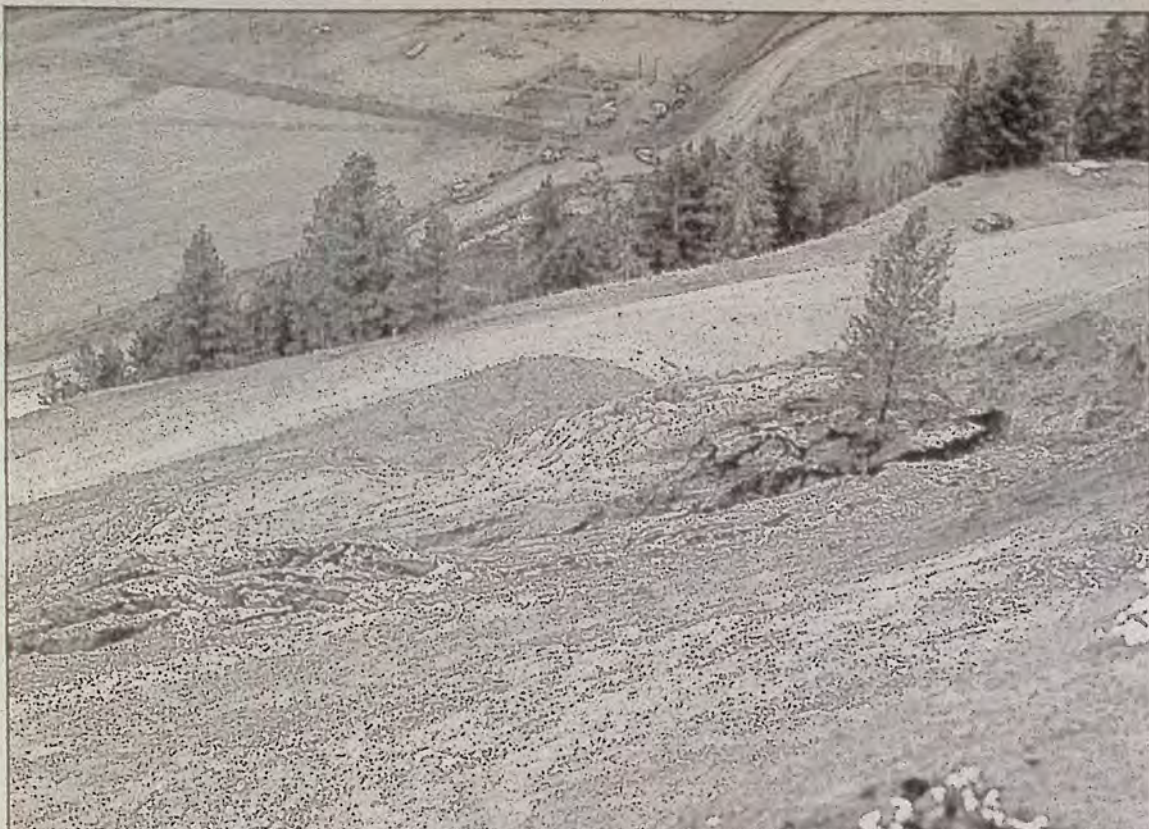
The upper embankment above the Coalmont Road at Peterson Bluffs began to slide on March 31. Construction was stopped pending observation for possible further slides. Note pine tree remains standing despite slippage.
