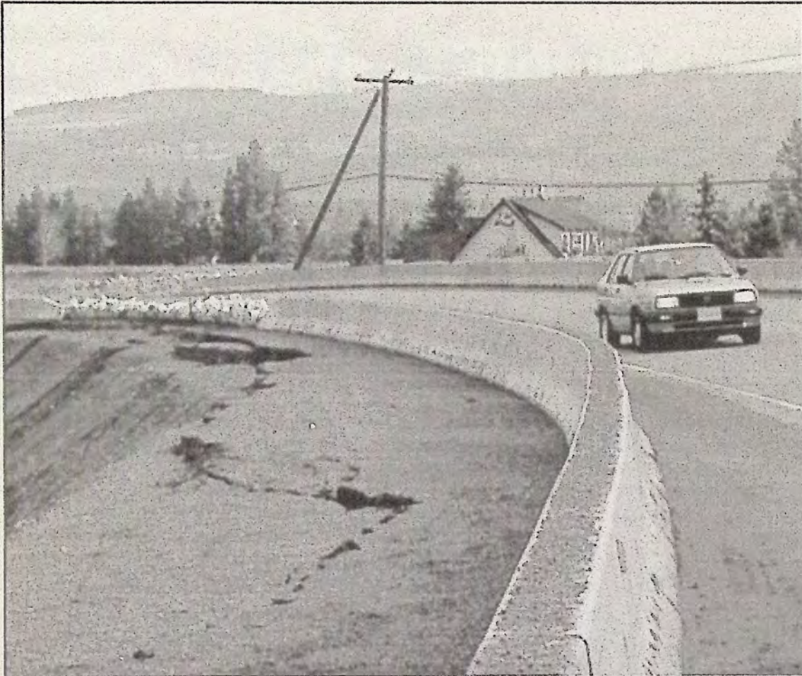
During the early morning hours of March 31, the slippage area 1 km west of downtown Princeton dropped approximately 40 cm (14 inches). Note white plastic bags filled with sand have been placed to alert motorists.
