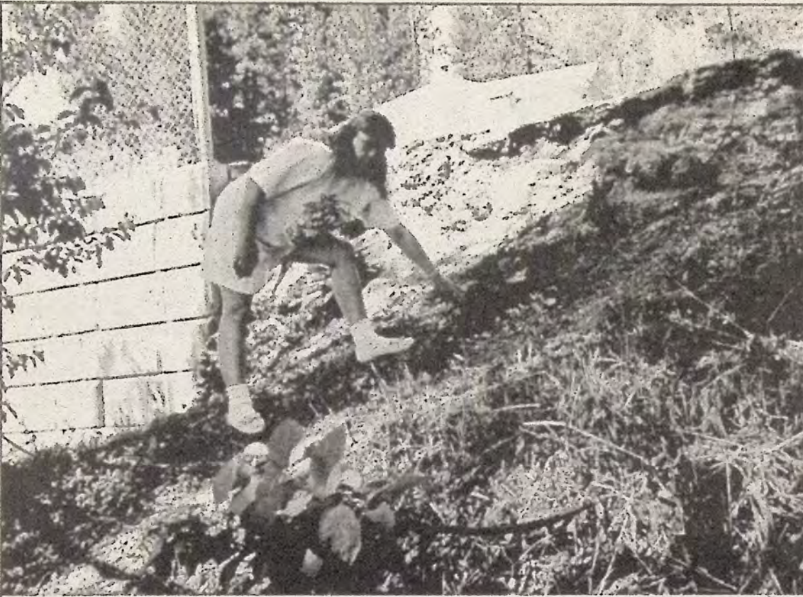
Diane Wanner points to a black chunk of asphalt fallen from Tulameen Road. Note ragged edge of asphalt to the right of the concrete retaining wall. The Wanners have objected strongly to the provincial government "devolving" road problems onto Princeton.
