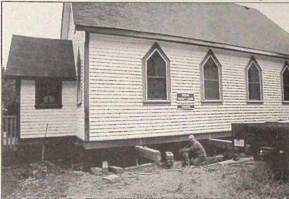
St. Paul's -St. Cuthbert's United Church had a wood foundation. The foundation was rotting. The church has been raised and a concrete foundation is being poured.
