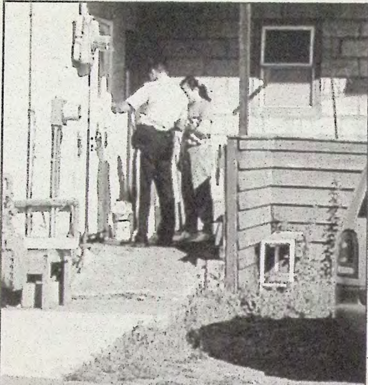
RCMP Constable Steve Barton examines the back door of the Leisure Inn where the lock was forced sometime during the night of July 23 - 24. Thieves took booze, cigarettes, prawns, chicken fingers, and money. Anyone having any information is asked to call Princeton RCMP at 295-6911.
