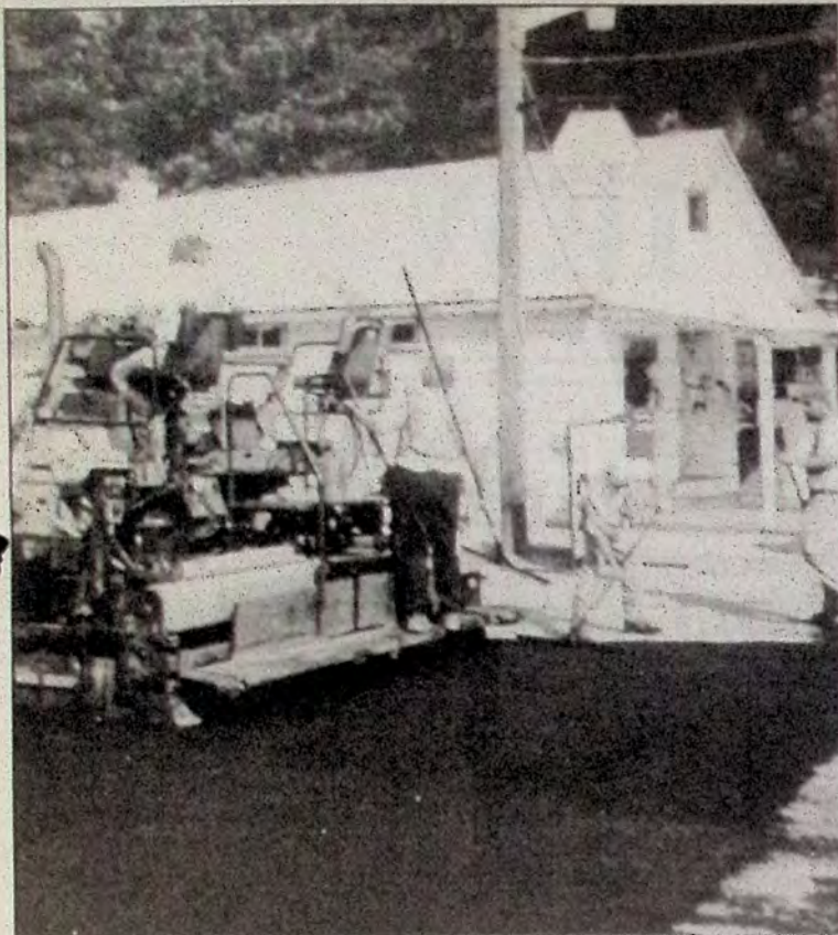
Downtown Tulameen is enjoying a face lift this summer. Above, the crew works on the main intersection in front of Tulameen Trading Post located in the heart of downtown Tulameen.
