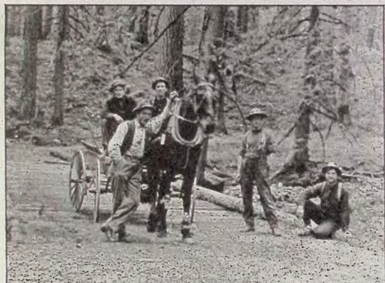
The photo above is a snapshot of the crew building the road between Port Alice and Port Hardy on Vancouver Island circa 1910. Note the outstanding bridge they built.
