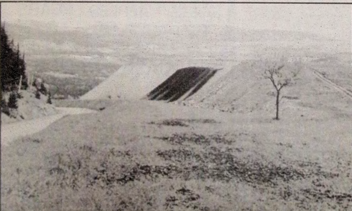
Revegetation of Steep Slopes at Similco - June 10/96 Steep waste dump slopes are another reclamation challenge at many mines. We are testing a variety of methods of applying biosolids to steep mine slopes. Background shows newly applied slope with recently fertilized highway berm in the foreground.
