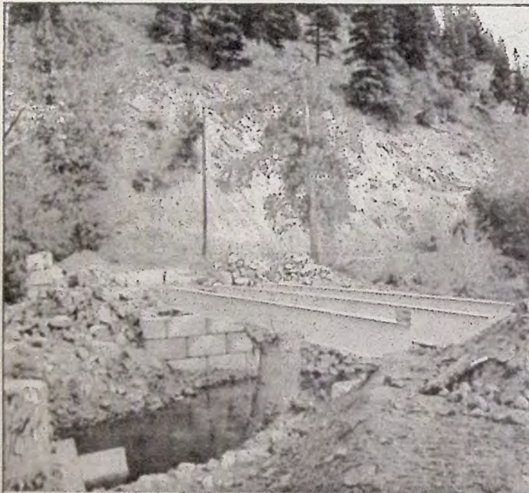
The new bridge rests on three large steel girders placed on concrete block foundation. The bridge offers an alternative crossing over Otter Creek and may become extremely important in floodwater conditions.
