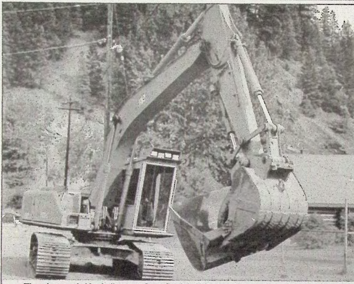
There is a new bridge built across Otter Creek in Tulameen. Above, Doug Miller operates the scoop used to excavate the dirt from the construction area.
