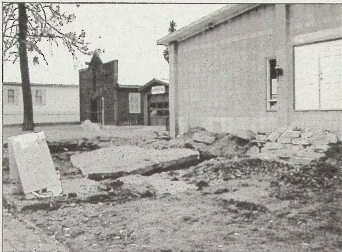
This big mess in front of the Library/Museum building is the first step in the exterior renovations to the building which will offer wheelchair access in the future.
