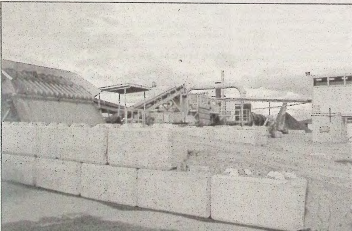
This is the Envirogreen Technologies site where hydrocarbon contamination is cleaned out of soil. The photo above shows conveyor leading to the heating unit and the fine particle return pipe, the hot air release stacks and at right the control room.
