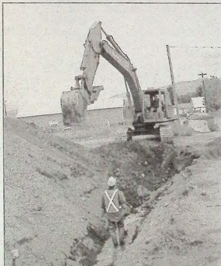
A new water main is going to the Similkameen Avenue area. Above, Ross Ferguson operates backhoe along Burton Avenue digging the trench for the new line which will loop the west end of town. That end of town was without looping since the embankment behind the Mohawk station collapsed three years ago. The person standing in the trench is town crew member Len Liberatore.
