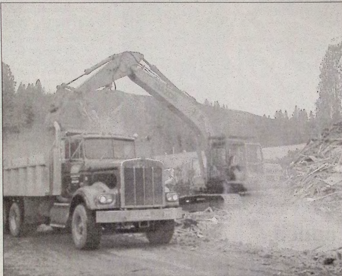
Contractors demolished houses along Burton Avenue last week as part of the effort to reclaim land contaminated by petroleum products migrating through the soil. The houses were condemned when residents smelled gasoline. The petroleum company purchased the houses from the owners.
