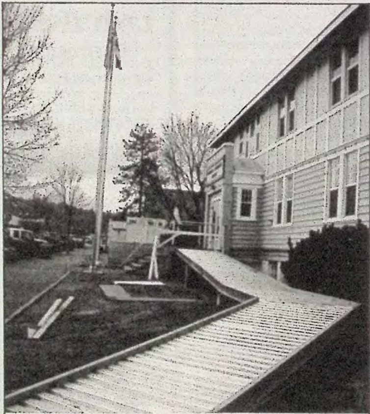
New concrete steps and a wheel chair access ramp are nearing completion at the Court House in Princeton. The work is being done by John Bachelder Construction.
