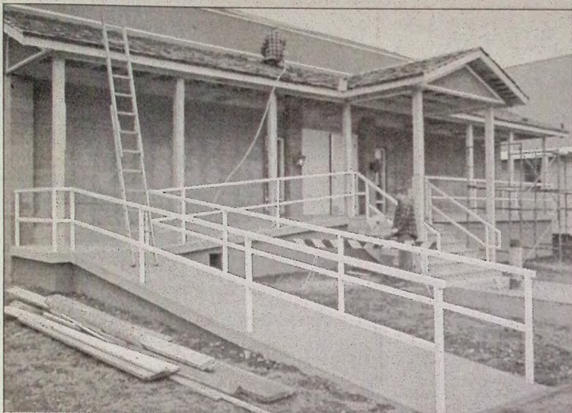
The new porch and ramp at Princeton Public Library and museum adds a whole new look to building. The attractive rose colored stucco adds a nice touch of color, but there is not enough money in the Town kitty to paint the grey brick.
