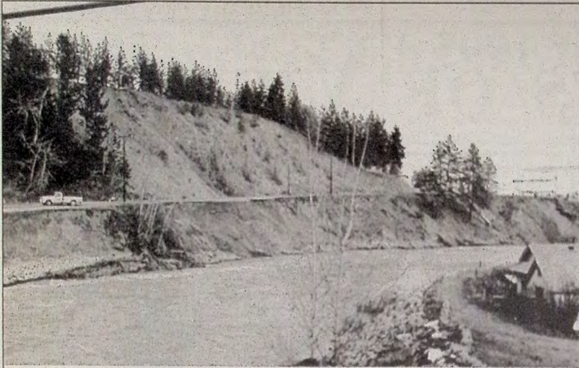
After the water went down following the flood of '95, the damage to the road leading from the wooden bridge to Riverside Intermediate became obvious.
