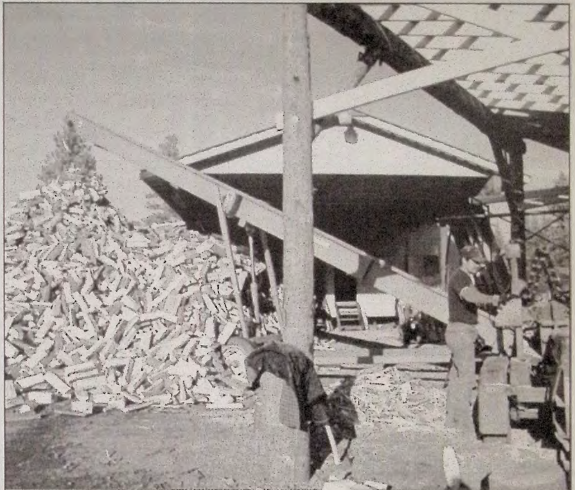
SBC Firemaster is back up to 75 - 80 per cent production after a four-week rebuilding process following the fire on October 15. This is Firemaster's busiest time of year and owner Wayne Wiren says his employees will be working extra hours to meet the demand for Firemaster's product.
