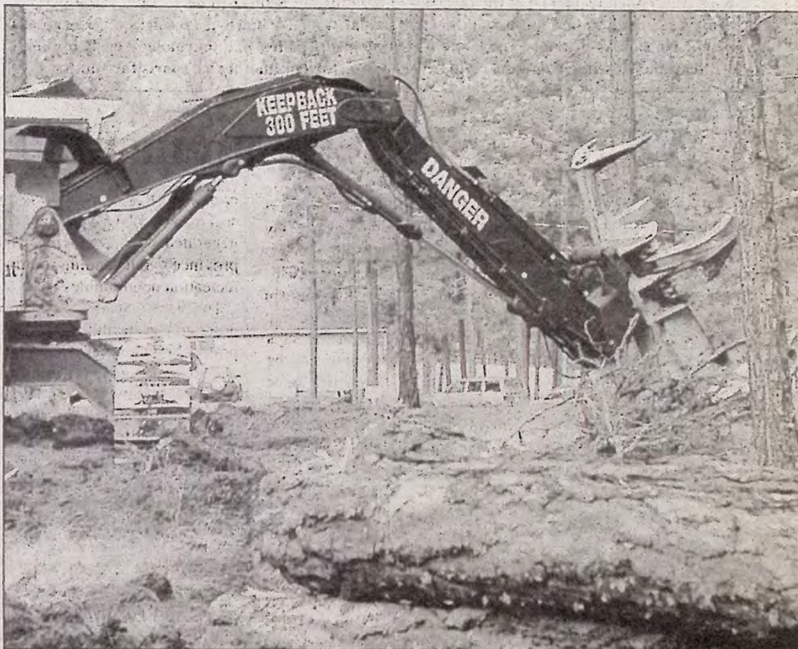
Work began in earnest last week on the golf course expansion. Loggers began clearing the jack pine from the path of future golf balls. Above, a feller-buncher is used to cut and clear the timber. A pile of logs in the foreground shows the neat efficiency of the operation.
