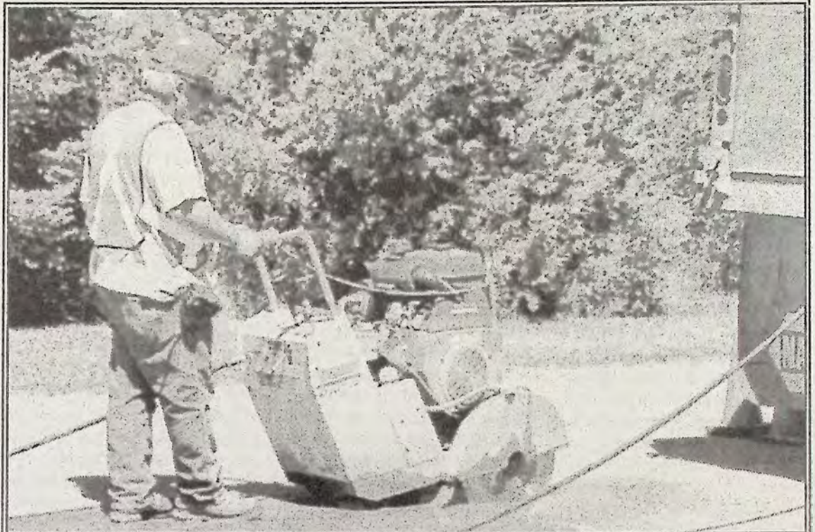
Eugene Deschamps does road repairs on 11th Avenue in Keremeos as part of the $14,555 Keremeos Village will spend this summer on road maintenance.
