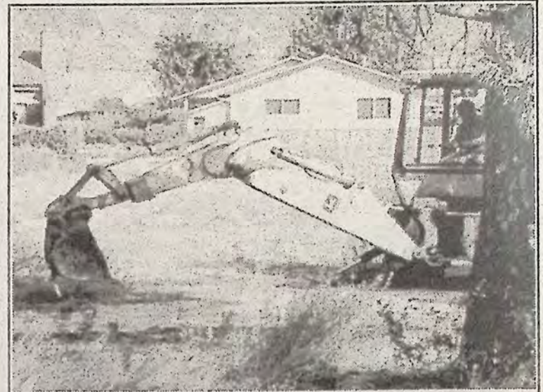
Front end loader digs trench along pathway to put cedar edging in place at Keremeos Riparian Park.
