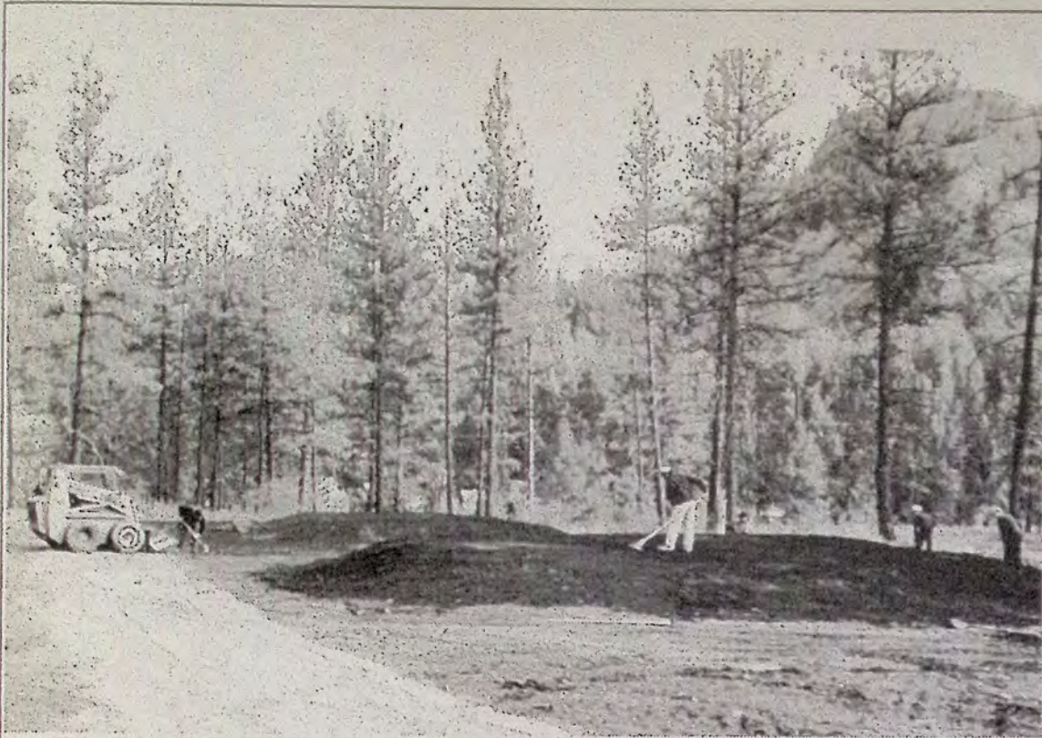
Work continues on the new nine holes of Princeton golf course. It is hard for most people to imagine the amount of work that has gone into the new development. Some of it is careful manual labour with rake and shovel, as shown above.
