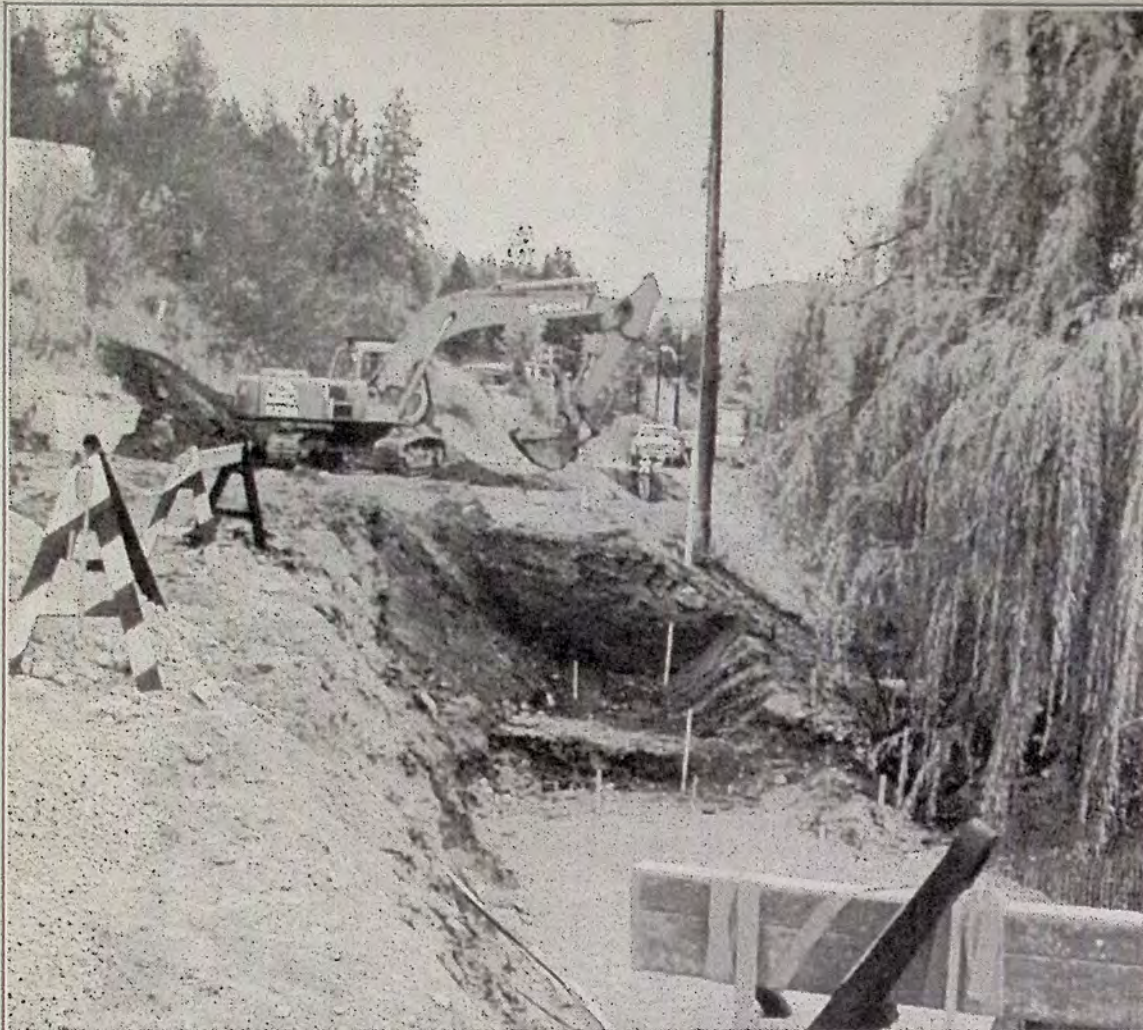
Tulameen Avenue was detoured all last week as work began on a retaining wall behind houses on Luard Avenue after a campaign launched by Ken and Diane Wanner, and taken up by Town Council, who refused to accept responsibility for the road until improvements were made. The road bed was collapsing and revealed burlap sacks filled with gravel holding up the asphalt.
