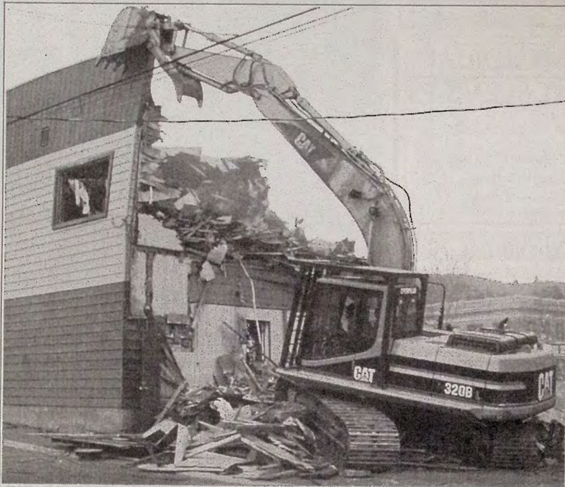
Edgar Minshull begins tearing apart the 1912 building that has housed the Spafford clothing store, Dorothy's fabric shop and Robert Wicks' law office. The building was purchased by Princeton Light and Power and slated for renovation. The old building proved to be beyond reclaiming. A new building, of very similar appearance, will take its place. The demolition drew a crowd.
