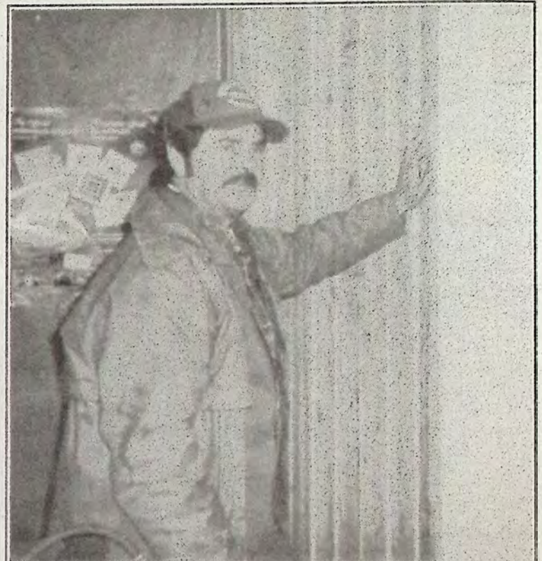
Tulameen Trading Post is undergoing some major renovations these days. Above, owner Bill Brent puts up a new look for the wall. Bill and Nola's steady customers find something new at every coffee break these days. Photo by Joe Schwarz.
