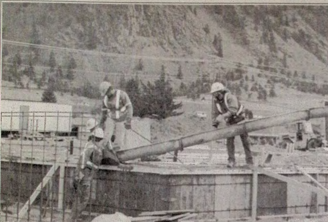
On March 8, the new South Similkameen Health Centre began to take shape as the construction crew fills foundation forms with concrete. Photo by Laurel Arnold.
