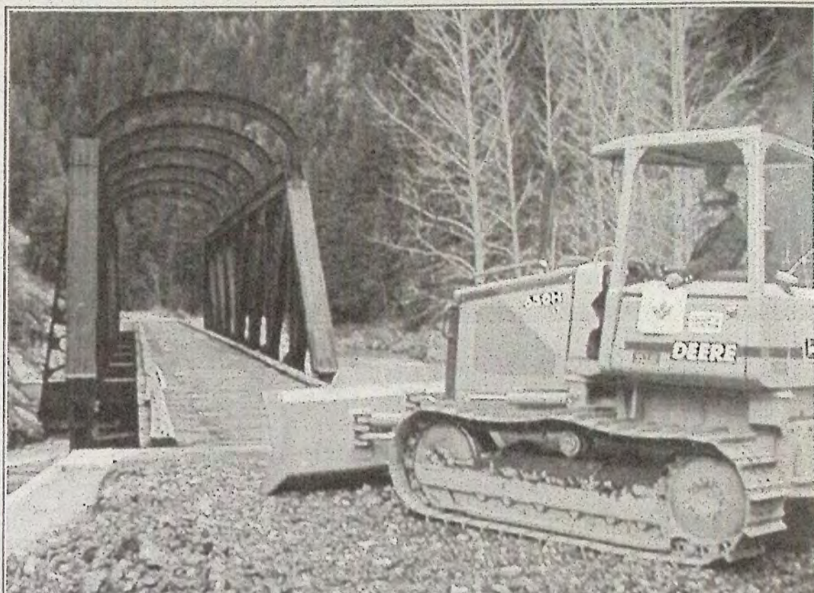
Ed Forde persuaded Coast Tractor of Westbank to donate the use of this John Deere Crawler 2000 for a week. Then Ed donated his time to work on the trail. He levelled, raised, lowered and repaired the entire Trans Canada Trail from Coalmont to Princeton! Last weekend, volunteer crews did a great job in the downtown portion of the trail, placing logs, raking, shovelling and doing clean-up.
