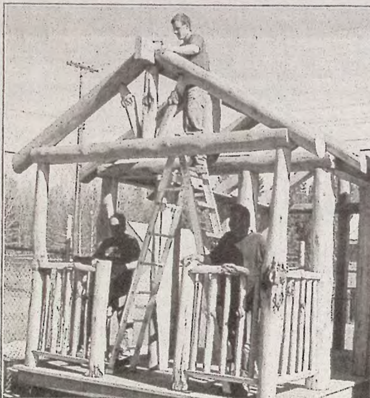
Princeton Post and Beam built a sample display cabin at Irvy Bird last week. Jimmy Parks is shown working at the top, and partners John Whitfield and Dave Isaacson in the shadows on the cabin front porch. These cabins are made from wood that would go to waste. A cabin the size shown would take two days to build. A larger cabin would require ten days. Parts are pre-cut. Average cost is $55/sq.ft. Modular walls fit into place easily.
