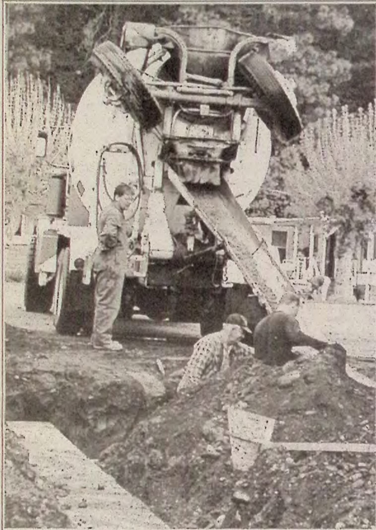
It was a historic moment for members of Princeton's Museum Society on May 9 as they watched the first pour of concrete for the foundation of the Pollard Wing which is scheduled for completion on July 15. The addition to the museum will house the impressive fossil collection assembled by the late Joe Pollard.
