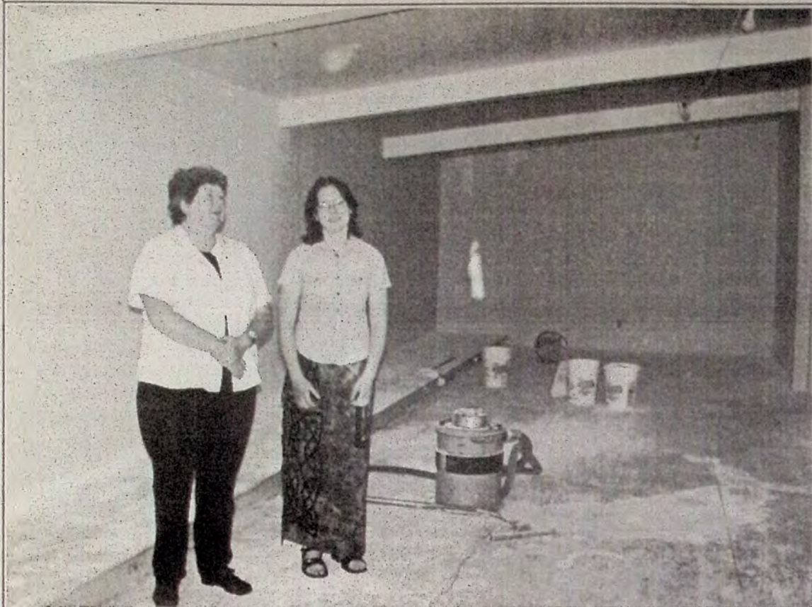
Rosemary Doughty, President of Princeton Museum Society, and museum attendant Meghan Barrie are shown in the almost complete Pollard Wing of the museum. Only half the length of the addition is shown in this photo. Drywalling is finished, and carpets are coming.
