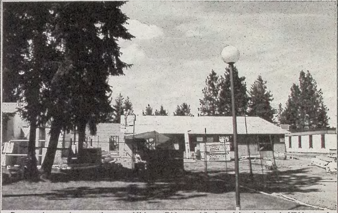
Construction continues on the new addition to Ridgewood Lodge, giving the hospital/Ridgewood complex a whole new look.
