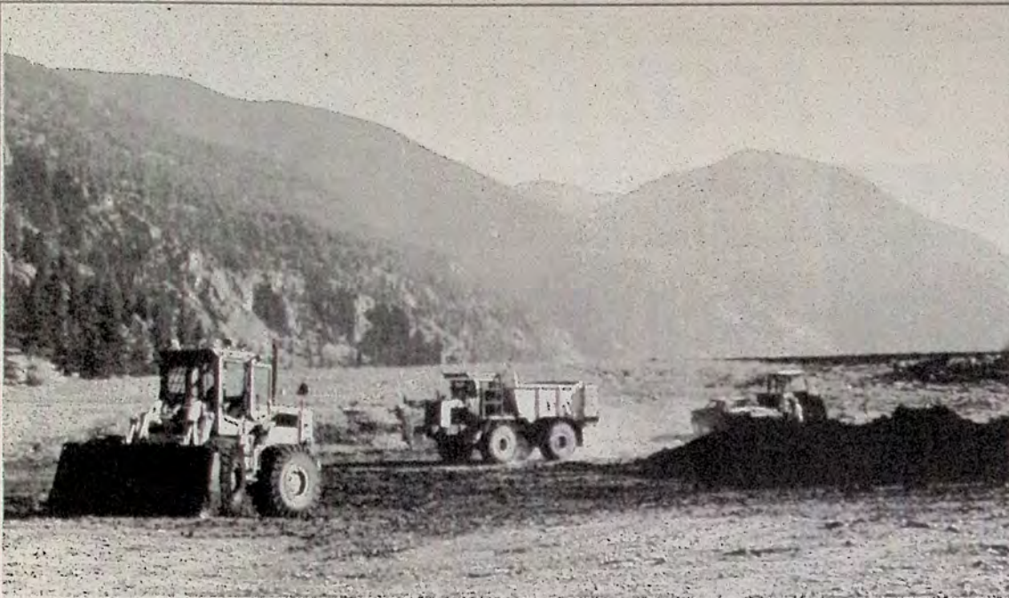
Wayne Crimmons and crew should be finished the reclamation project at Hedley at the end of the month. GVRD sees the former heap leaching site as a "showcase" project for next spring.
