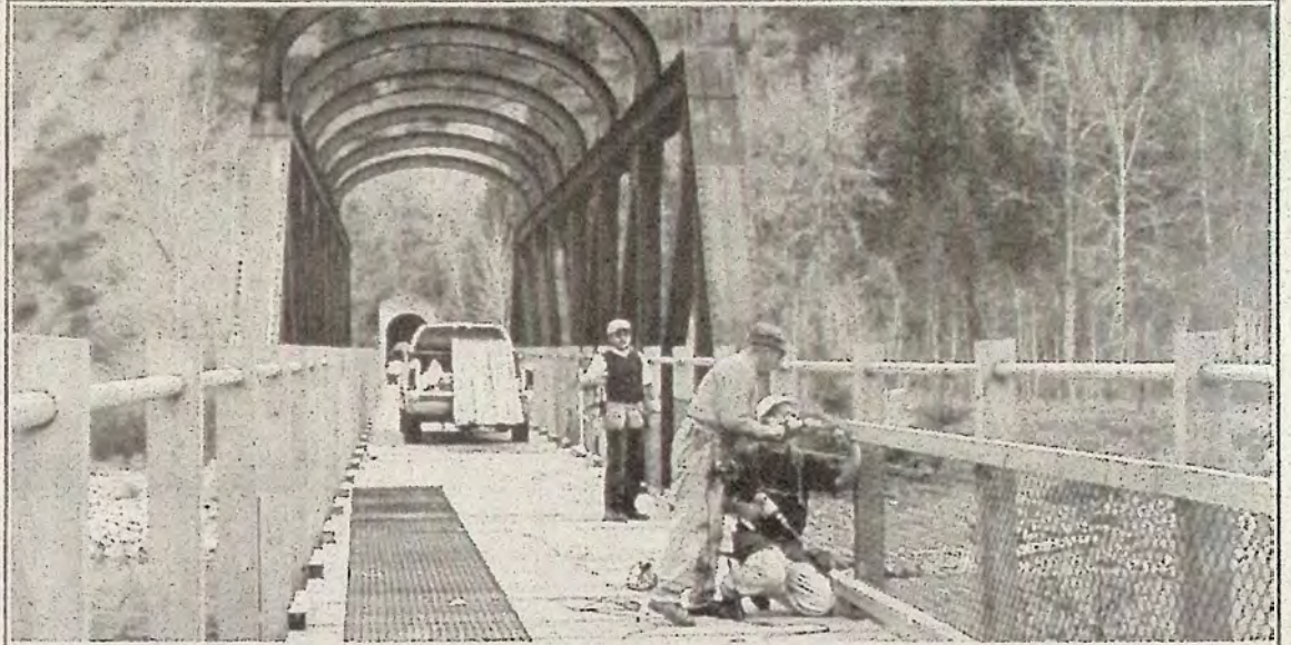
Cumming Construction is doing a great job of turning the trestle into a safe walkway. Above, Willi Drees, Tom Cumming and Shawn Hume put up safety wire to finish up the project.
