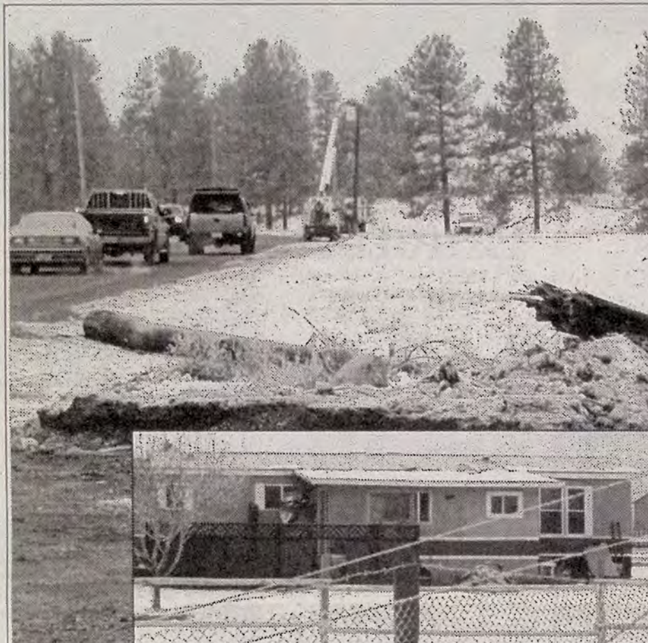
Princeton Light and Power repairs lines on Sunday morning. In the foreground is the pole snapped off when a truck careened into it. Lower right: the home of Ed and Sally Nault, showing the downed lines along the Highway 40 in front of their home. Damage to the Nault home will be evaluated this week.
