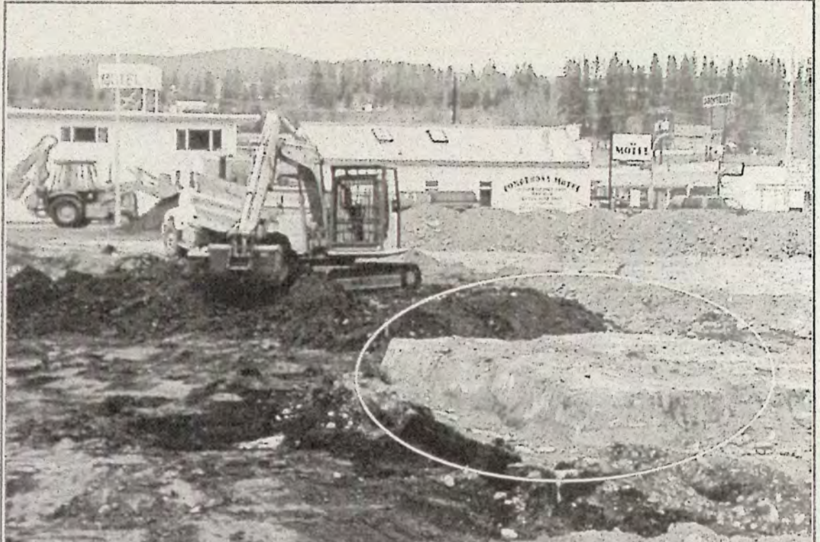
Construction began on the site of Valley First Credit Union's new building last week. One of the discoveries was a large concrete square not far beneath the surface (see white circle). Sidewalk superintendents speculated as to the purpose of the concrete, and all kinds of answers came to light, but none tells us exactly what it is. Reicherts, doing the work, have no idea what it is.
