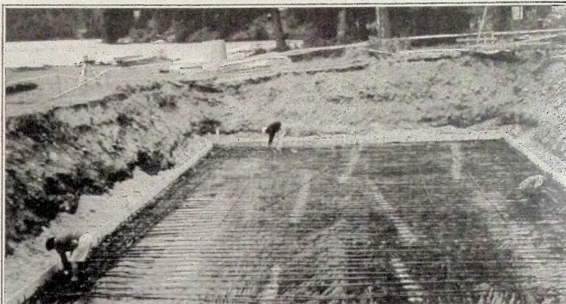
This is the new filtration tank for the modern water supply intake for Missezula Lake residents. The roof has been constructed now, and the final phase of construction is underway.
