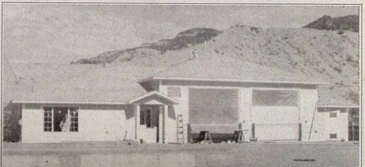
A great deal of progress is being made on the new ambulance station in Keremeos. No date has been set for the Grand Opening.
