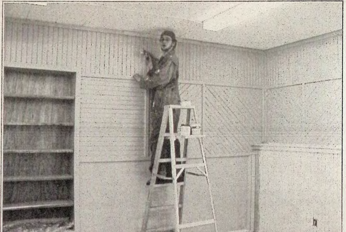
Claude Lalonde, above, is one of six Katimavik volunteers who worked hard at renovations to the basement of Victory Hall. Last week, volunteers painted old and new walls in deep gold and plum. The new carpets go in this week. The Employment Access Centre is an exciting development.
