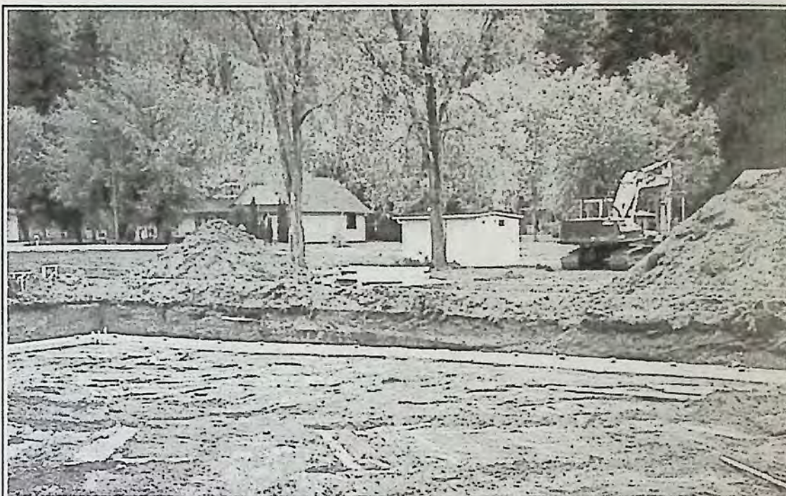
The first foundation for the new subdivision was laid last week, as shown above. The new subdivision marks another expansion in Keremeos of residential property.
