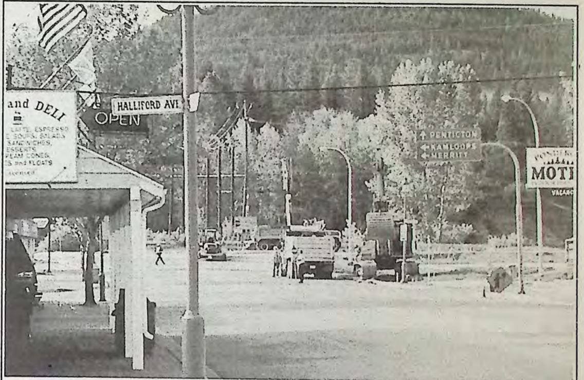
Work on Highway 3 approach to the new bridge meant tearing up part of Bridge Street in front of Valley First Credit Union building. Expect more traffic disruption in the next two weeks as the bridge nears completion. The intersection has been re-designed.
