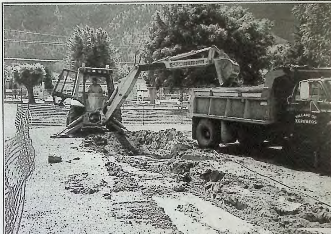
Village employee Eugene Deschamps digs up Memorial Park for new playground equipment. The old playground equipment will be installed at Pine Park.
