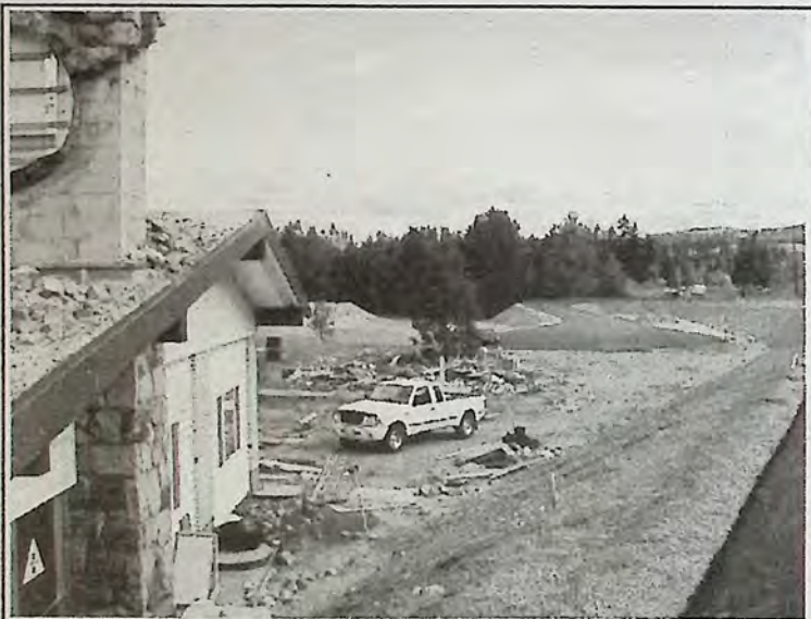
This is the old Chamber of Commerce building. Note where the highway encroaches on the building.
