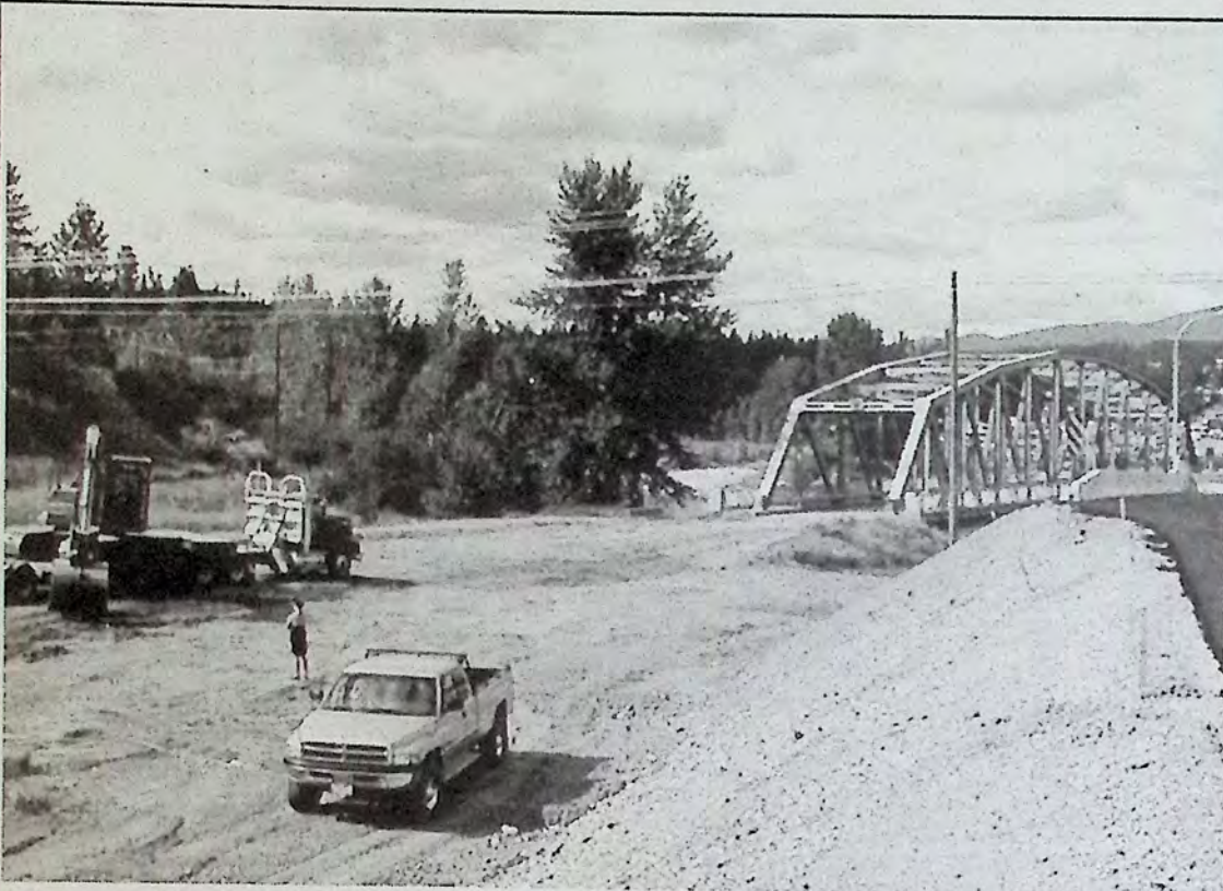
The asphalt has been removed from the old bridge approach as the process begins for the removal of the blue bridge. There is still a lot of work to be done before the bridge project is complete.
