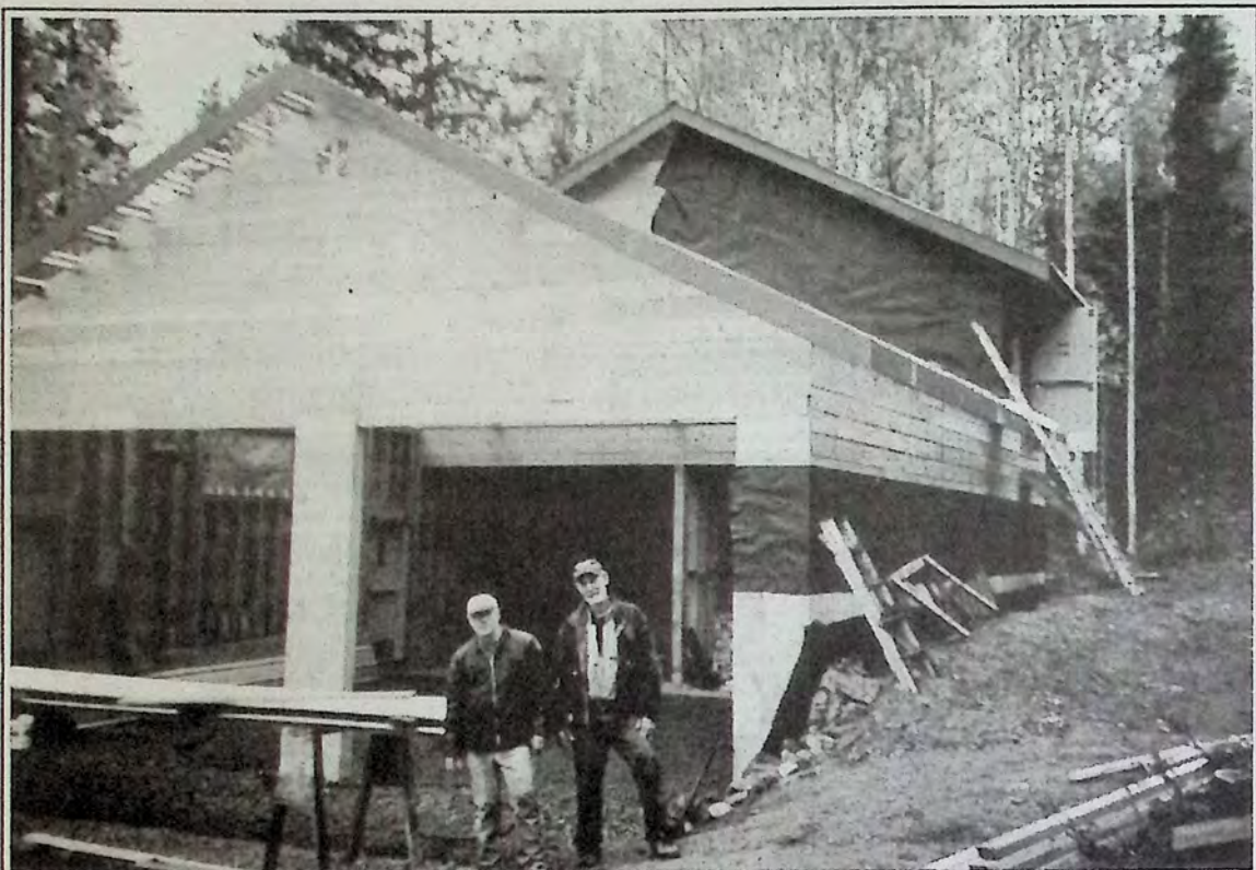
Dan Howland and Ray Callard stand in front of the new firehall serving Osprey Lake area.
