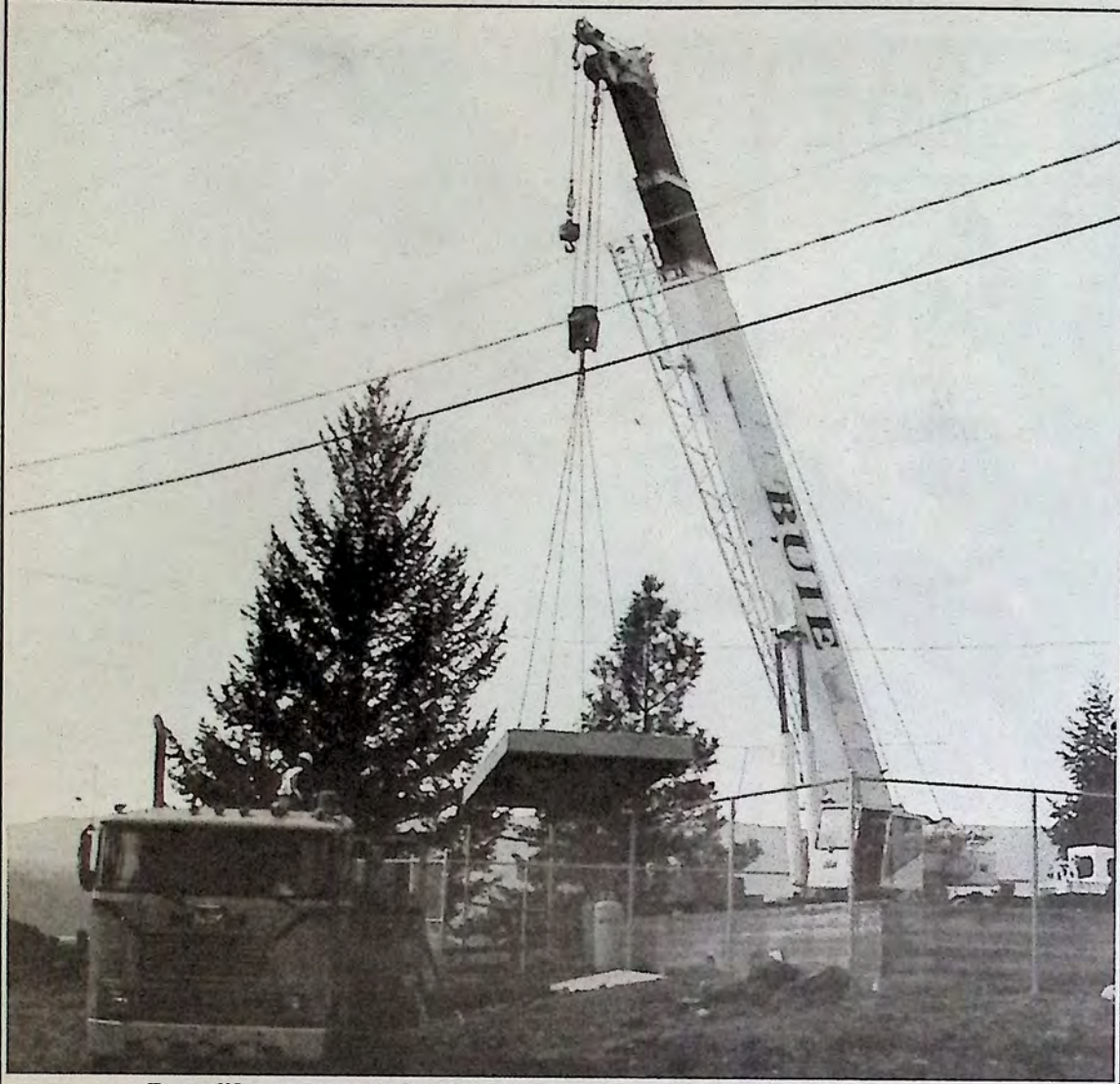
Crane lifts concrete roof section onto reservoir, working to avoid power lines.
