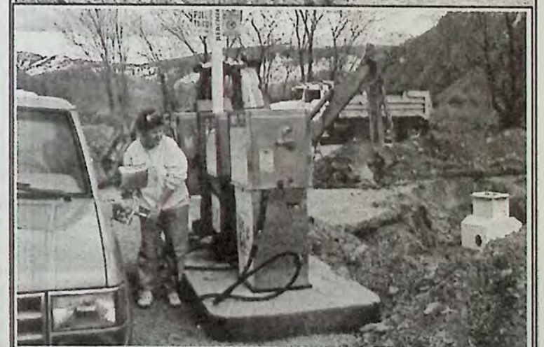
Pumping gas at Sportsman's Corner was a bit more difficult last week as renovations continued at that location. The popular stop has a brand-new building (top photo).
