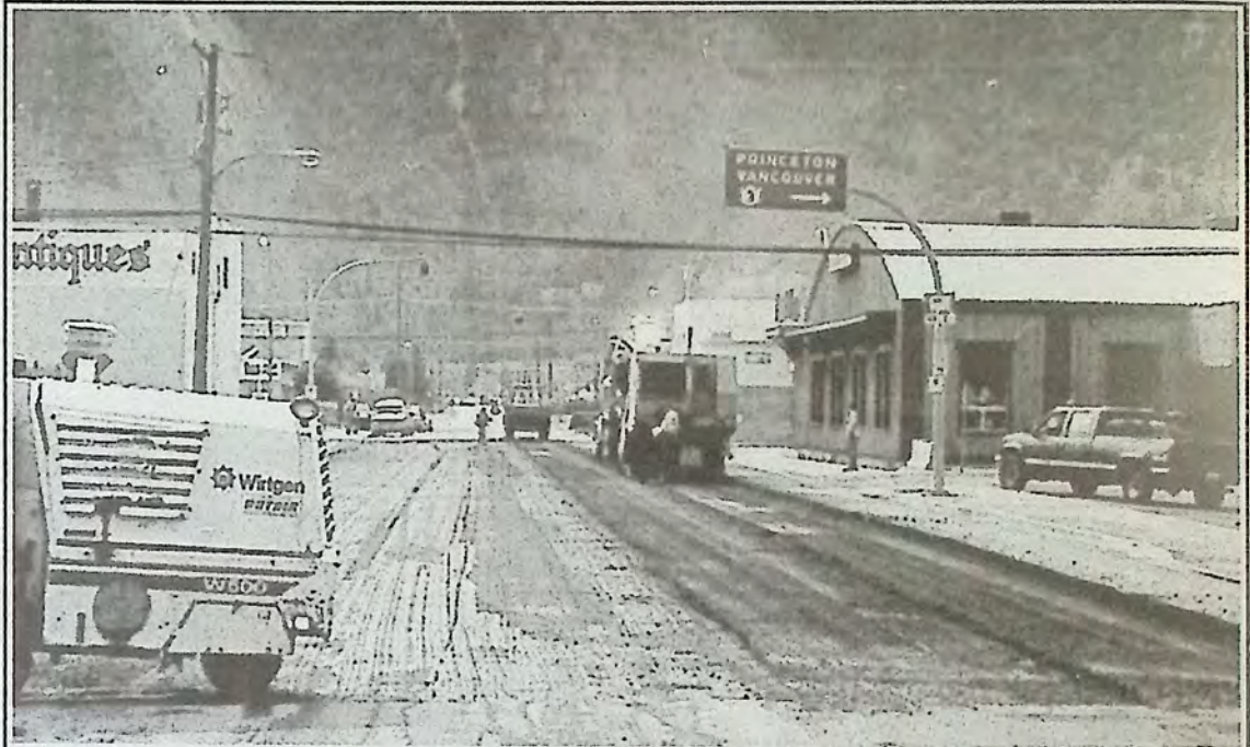
This was the view of downtown Keremeos last week as a major paving project on Highway 3 began. Single lane traffic and minor delays are to be expected for a few more weeks.
