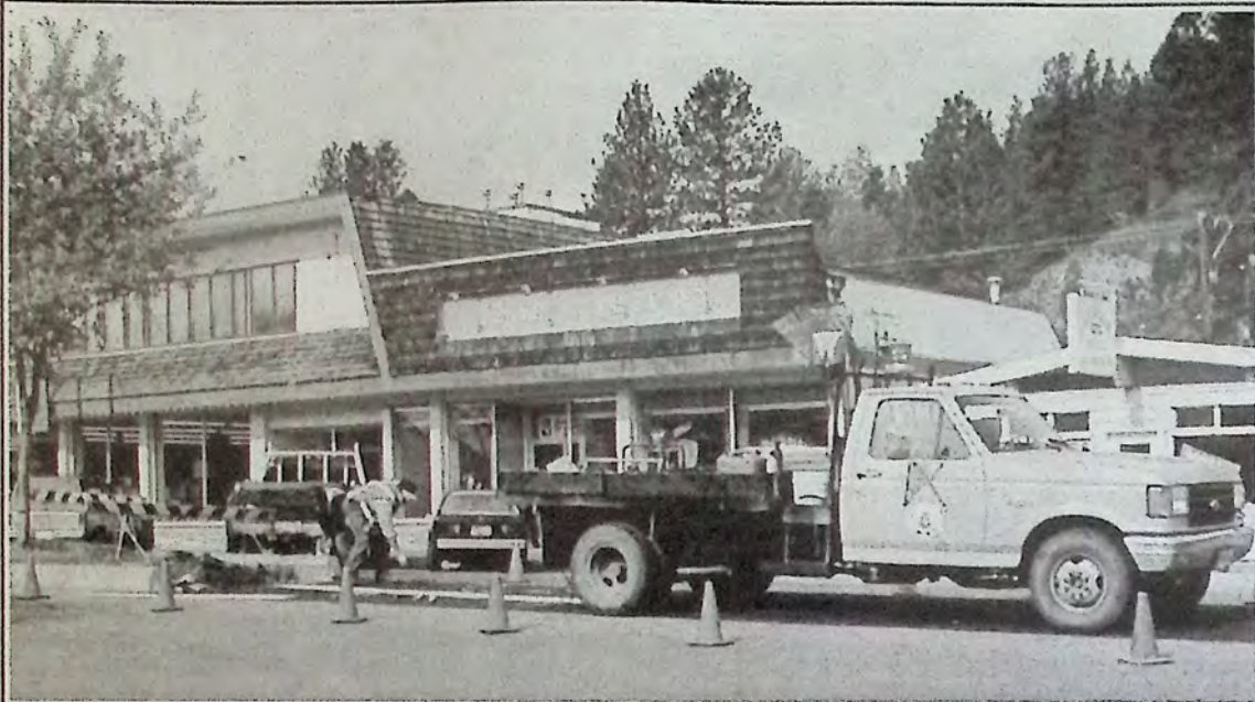
Town crew works on removing a section of the meridian on Vermilion Avenue to allow Best Western patrons to turn left when exiting the motel.
