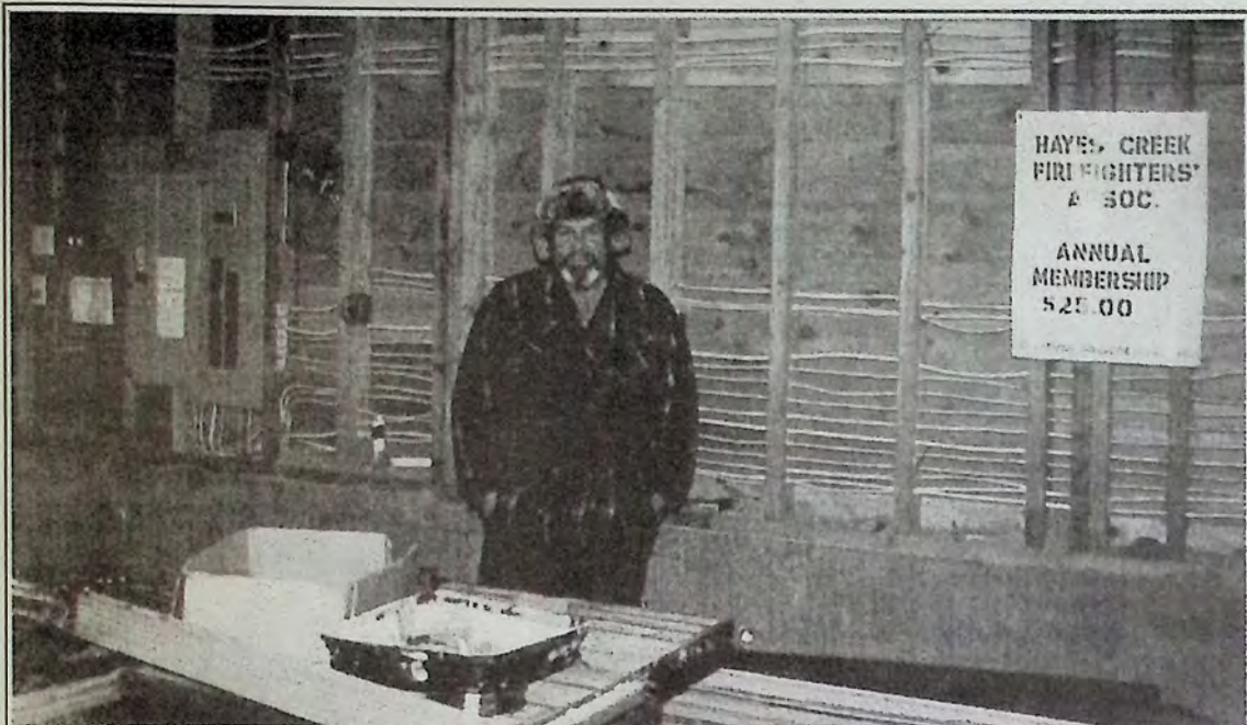
Brad Boyes, above, generously donated all of his time, skill and materials to put the electrical system in place in Hayes Creek Firehall last winter, and Directors and members could not thank him enough.
