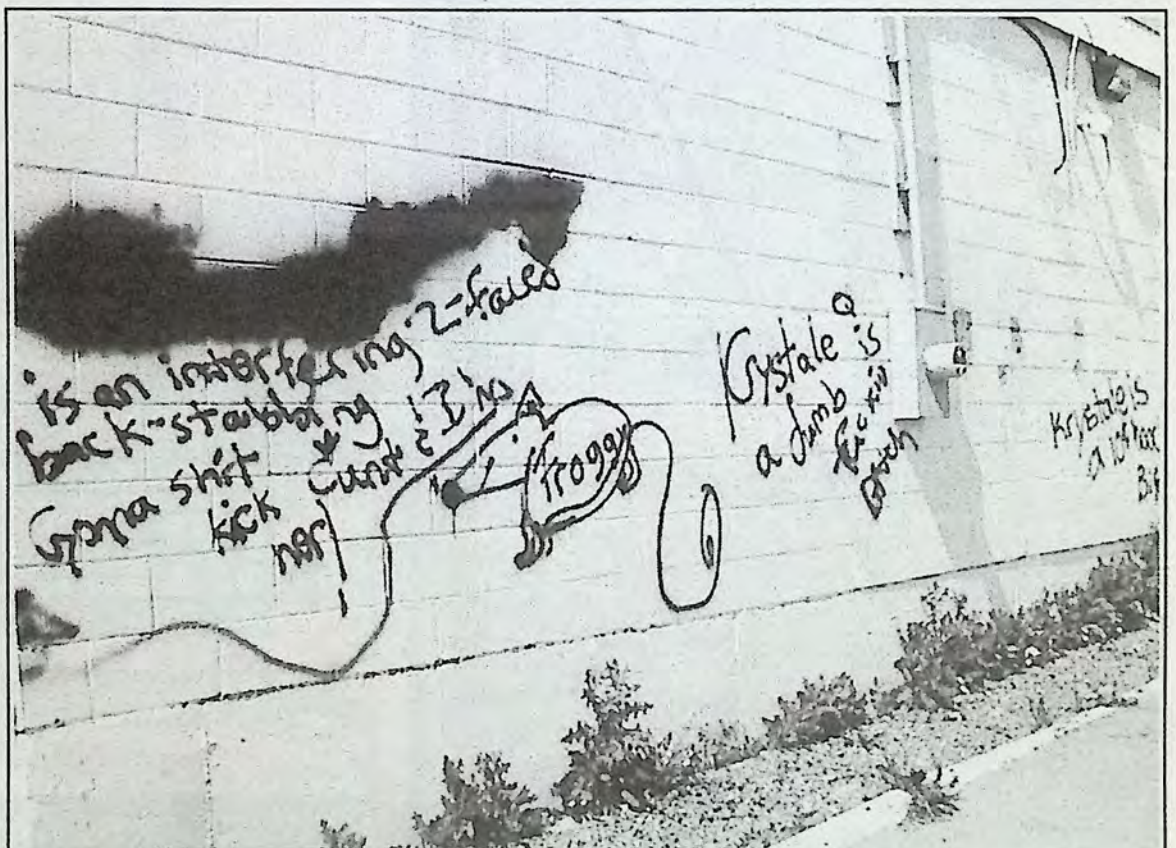
This is the mess at the back of the Lordco building. Purple spray paint was used to express a lot of ugly vindictiveness on buildings and vehicles. The total cost of clean-up will be very expensive.
