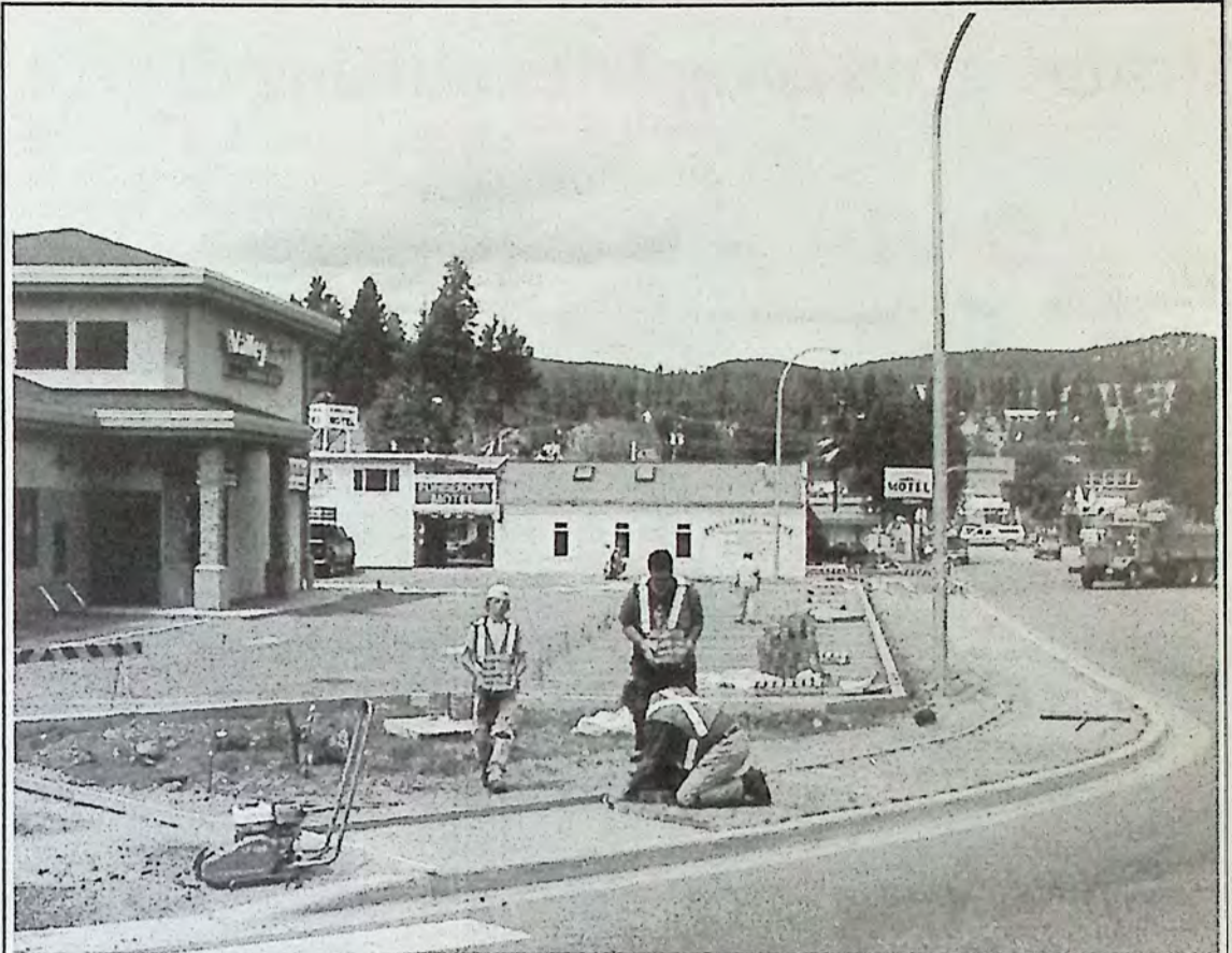
Henry Rykers shows student help how to lay a brick sidewalk. The new sidewalk was built last week to complete the project begun when the new Valley First building was constructed.
