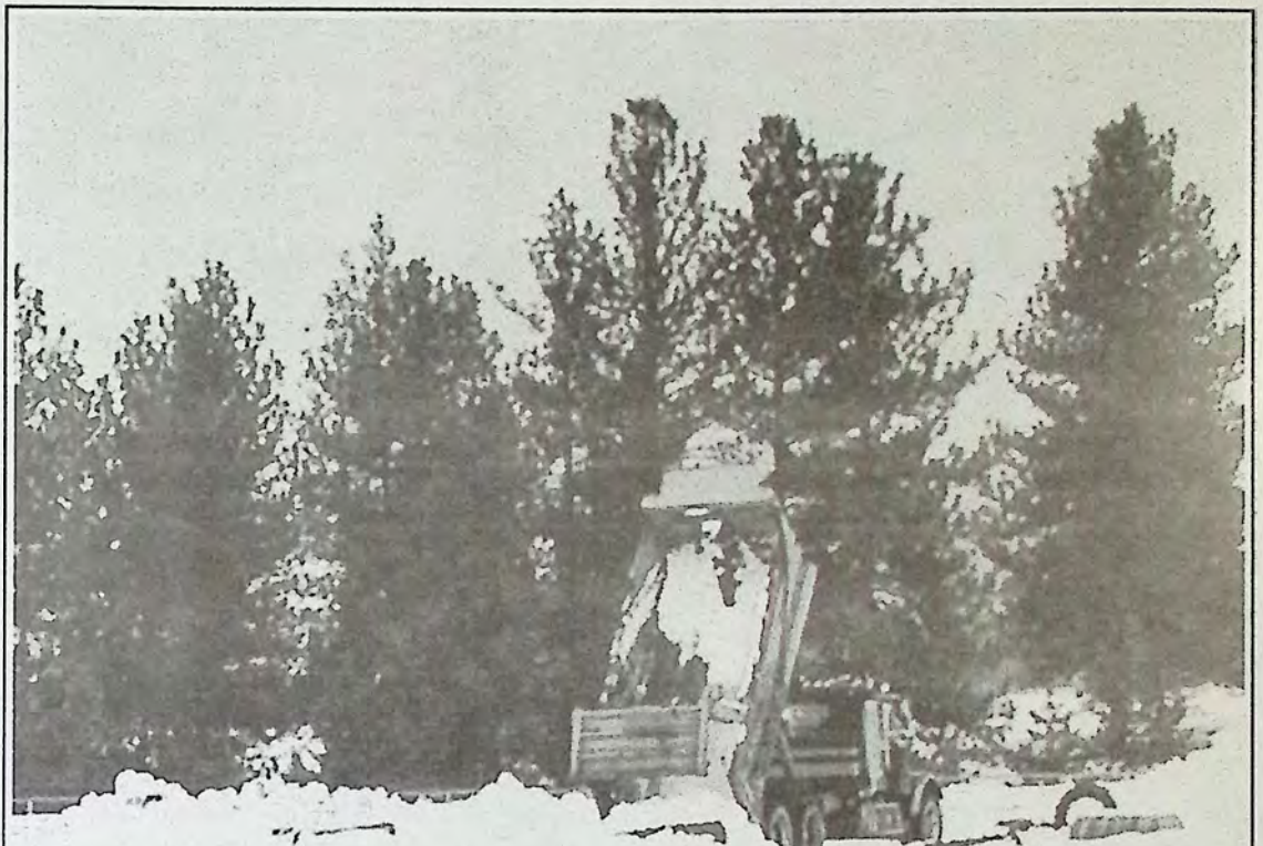
Princeton Redi-Mix truck dumps a load of snow on the tuff truck track at Princeton's exhibition grounds in preparation for Sno-X races. The jumps and bumps will be constructed prior to the race weekend. Rain hampered some work, and Timberline Cruisers hope for more snow.
