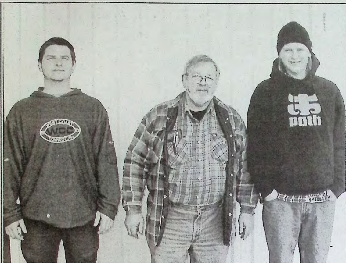
At Princeton Exhibition grounds, Peter Ruoss, center, has launched a work project with the help of Katimavik participants Jonathan Tremblay (left) and James O'Marra. These two young men worked with Ruoss last week on plumbing, putting hot water into the washrooms and refreshment booth. When that project is done, there are a lot more chores to do around PXA grounds. When this Katimavik group goes home, these two young men will know not only plumbing but a few other basic handyman skills. Their work is very much appreciated by members of the PXA, most of whom do not have the time to do all of the work required on the grounds.
