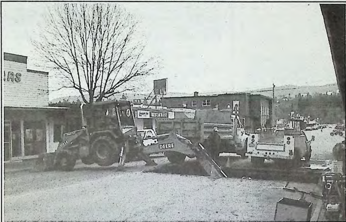
Water main repairs in downtown Princeton closed a portion of Bridge Street Tuesday morning.
