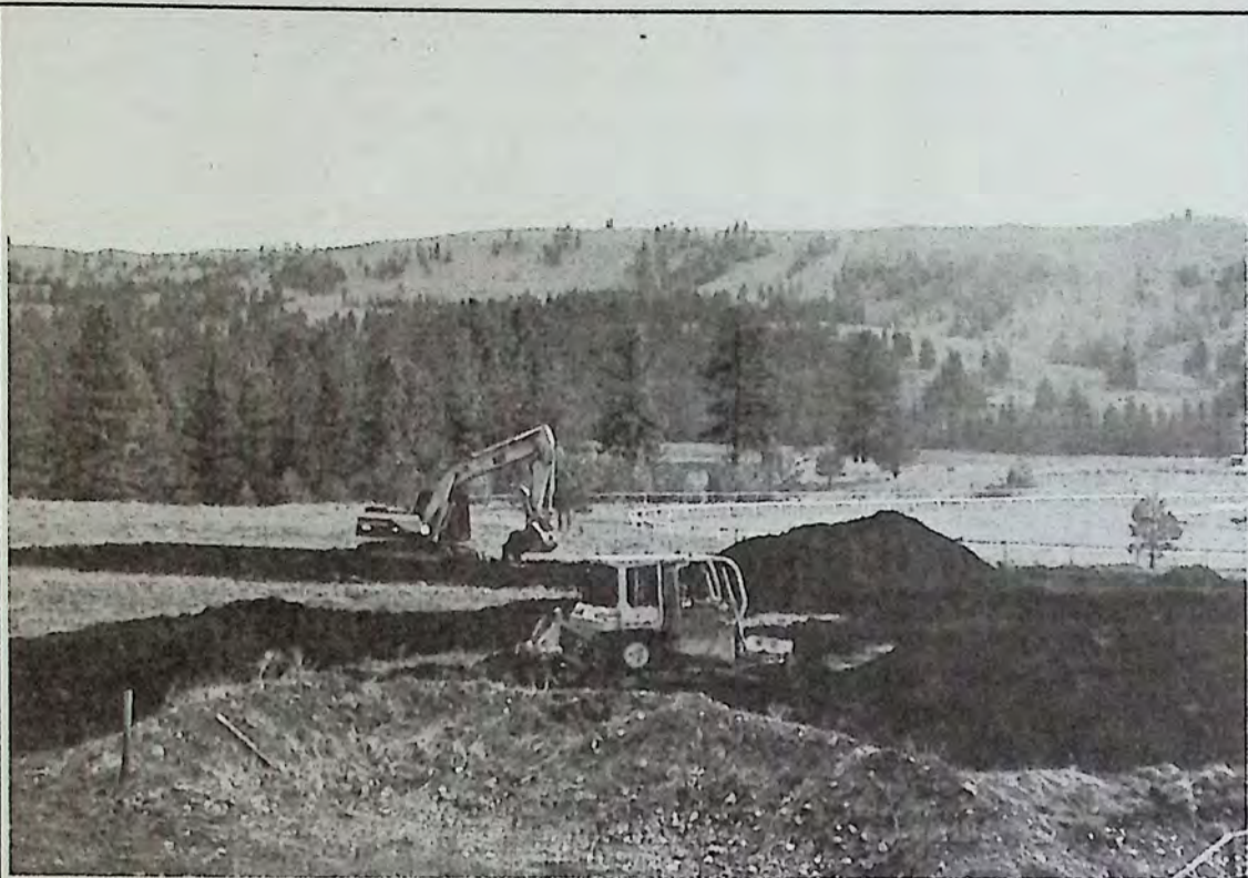
Construction at the west end of the racetrack puts motocross on a higher level bench.
