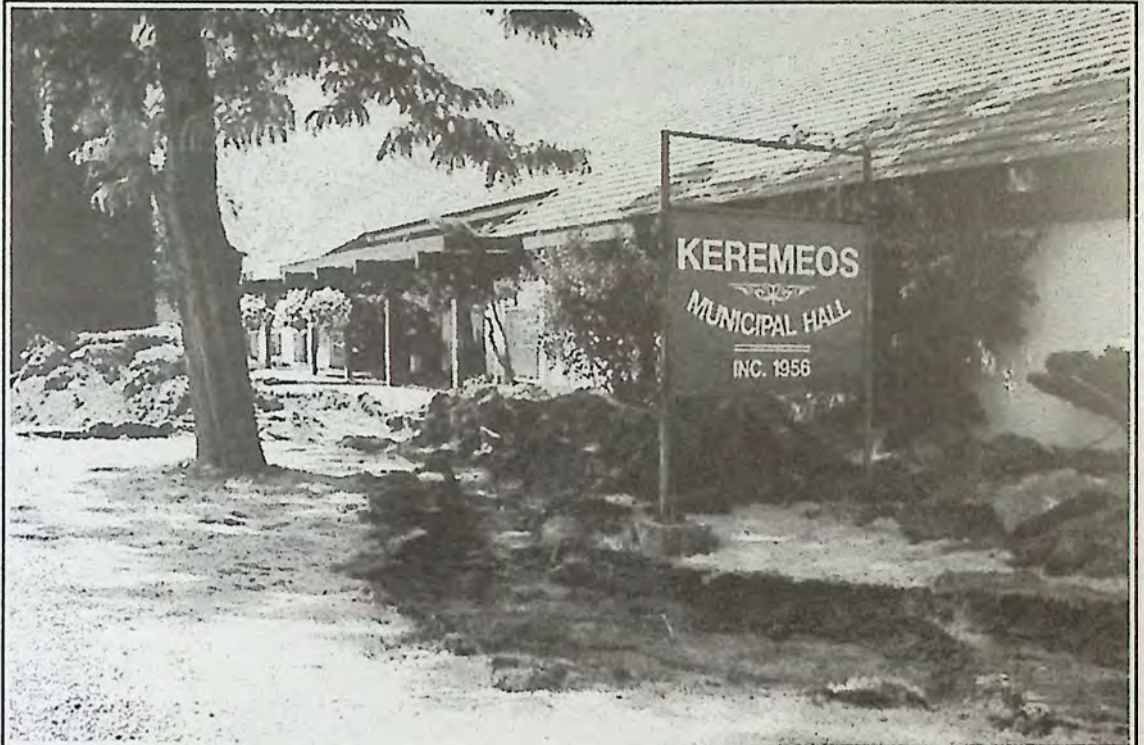
The lawn at Village Hall is totally dead and the area is being trenched for irrigation of the low water and low maintenance landscaping.
